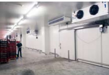
GGHN drycoolers in cold storage rooms
