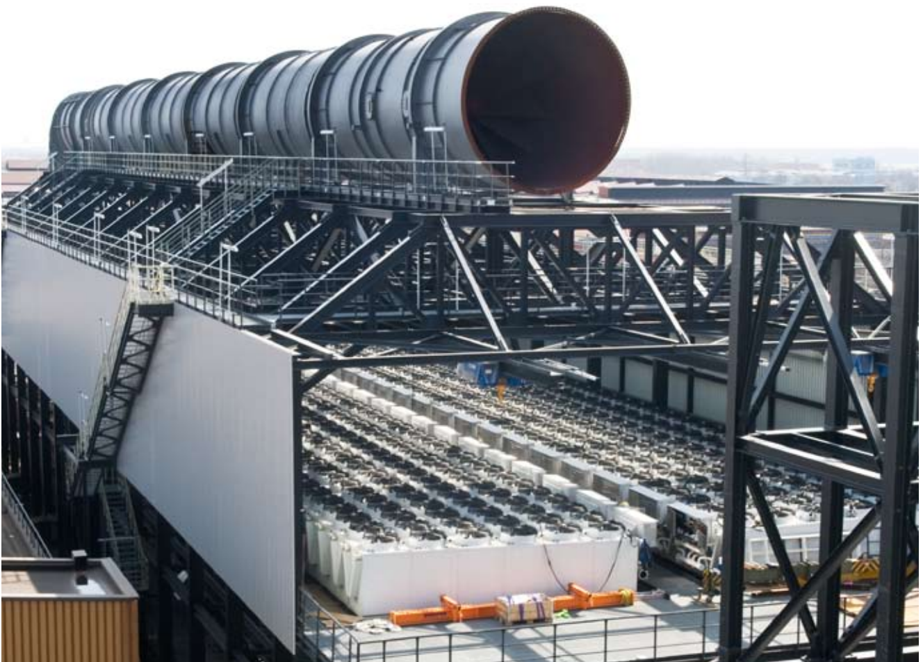
Güntner delivered a total of 64 drycoolers for this installation
