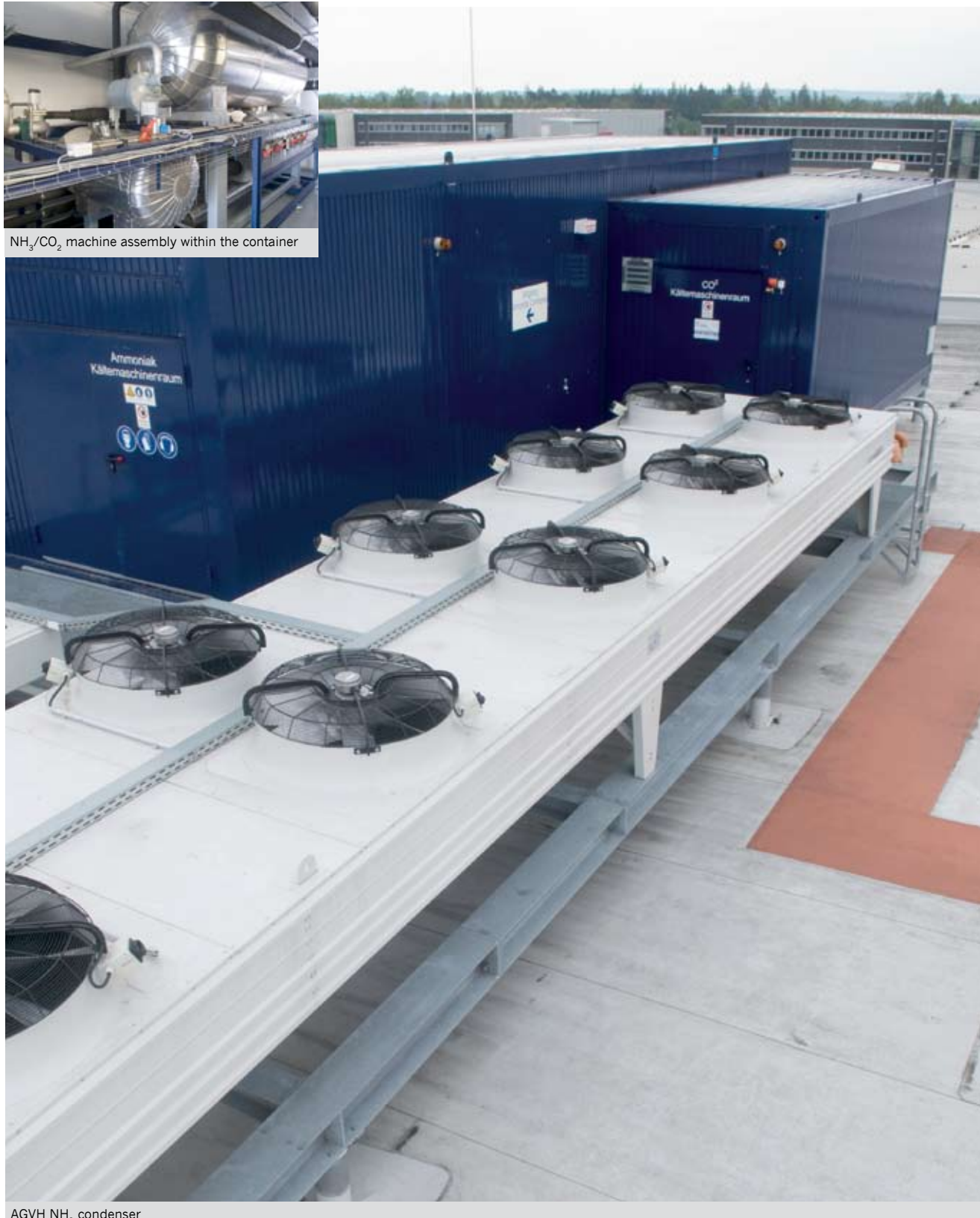
AGVH NH 3 condenser
