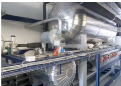
NH 3 /CO 2 machine assembly within the container
